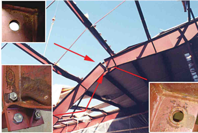
Fig. 1 — View of a bolted connection that failed as a result of snow loading on a roof.
